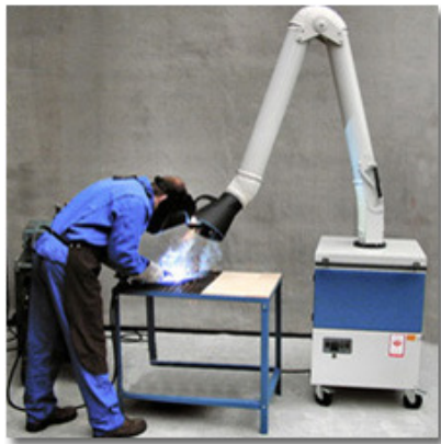
Extraction / ventilation system to ensure clean air supply
